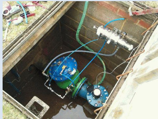
Aquai-mod (silver) installed alongside a pressure regulator valve.
